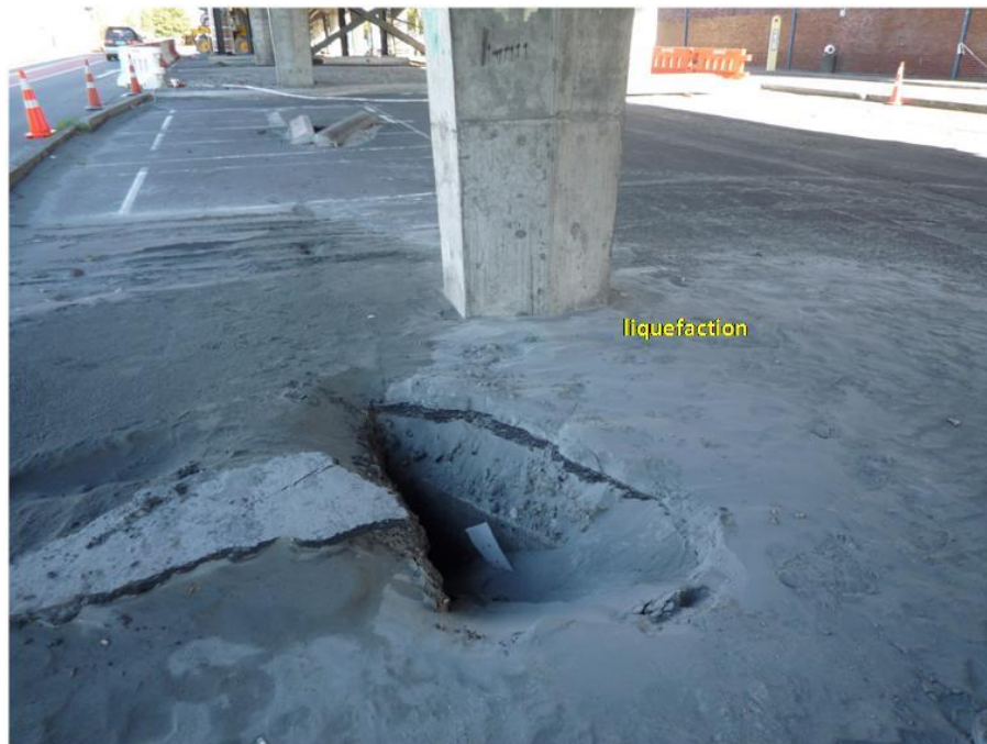
Figure 4.53. Sand-boils indicating liquefaction.
