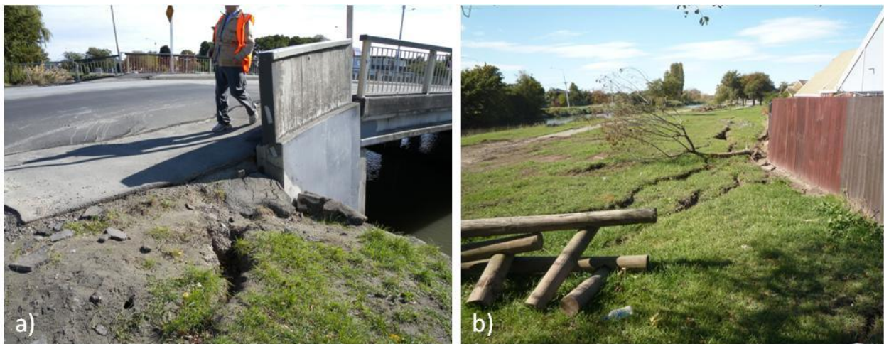
Figure 4.27. a) Back rotation of southern abutment of Avondale Bridge (B6 on map of Figure 4.1), cracks in the backfill, b) Large lateral spreading cracks in the south coast parallel to the river extending in a great distance at both sides of the southern abutment.
