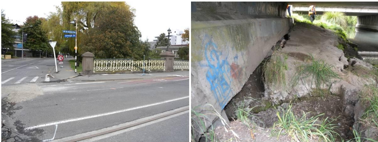
Figure 3.2. Bridge at Oxford Terrace (left) and rotated abutment of Fitzgerald bridge (right).
