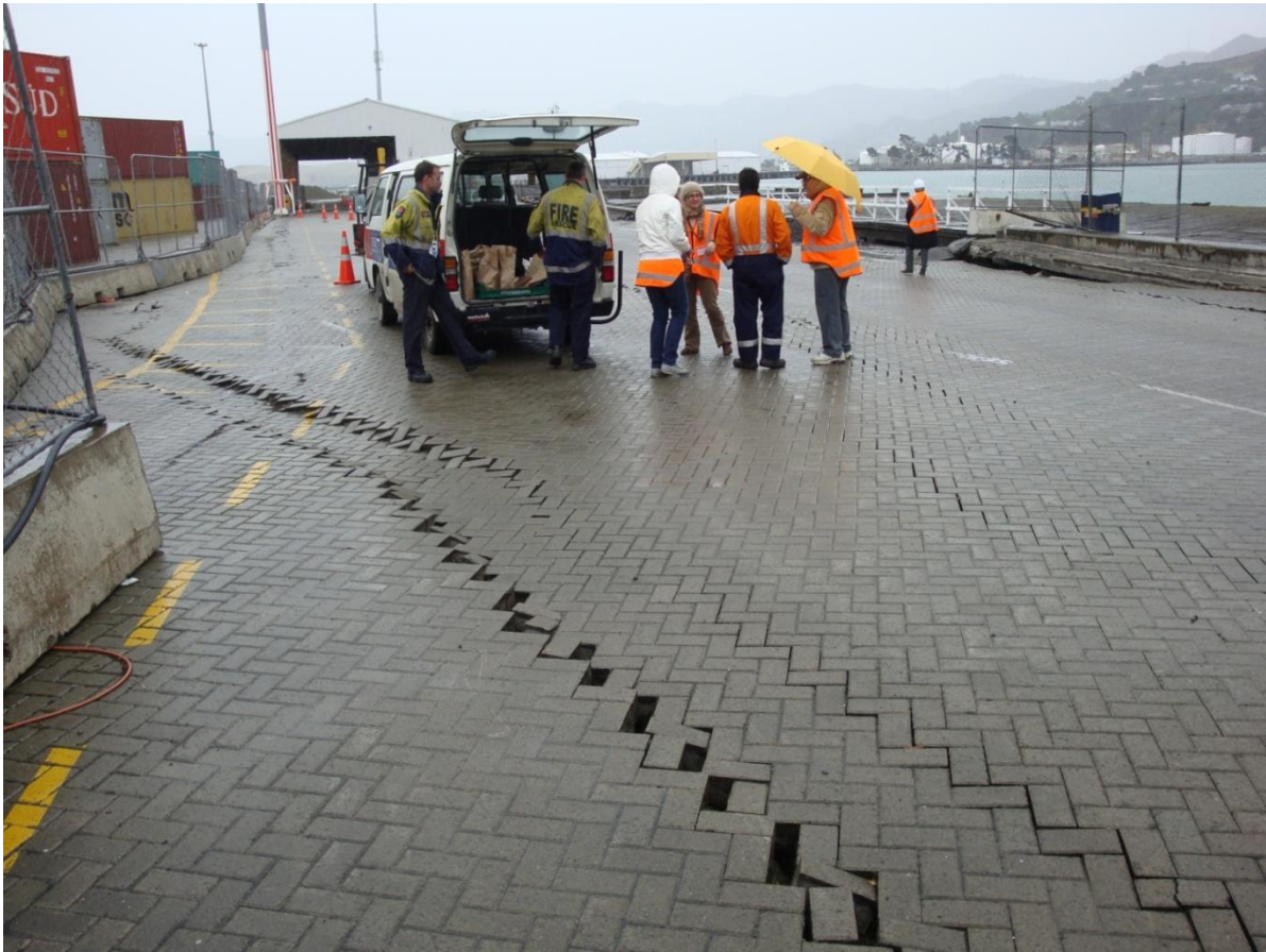
Figure 5.16. Cracks in the pavement due to lateral spreading continue to develop several meters behind the quay (site W2 pointed in the map of Figure 5.6).
