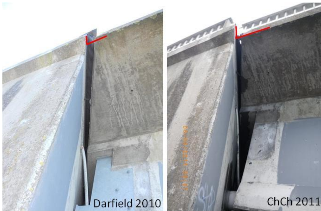
Figure 4.40. Western abutment of South Bridge Road Bridge (B8 on map of Figure 4.1). Slight differences between Darfield and Christchurch shaking events in terms of differential displacement of the abutment relative to the deck in the skew line direction. Source: NHP-Bridge Research Group.
