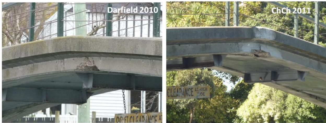
Figure 4.23. Snell Footbridge (B5 on map of Figure 4.1) after Christchurch earthquake. Comparison of damage between Darfield and Christchurch shaking events. The cracks have widened and extended at the mid-point. Source: NHP- Bridge Research Group.
