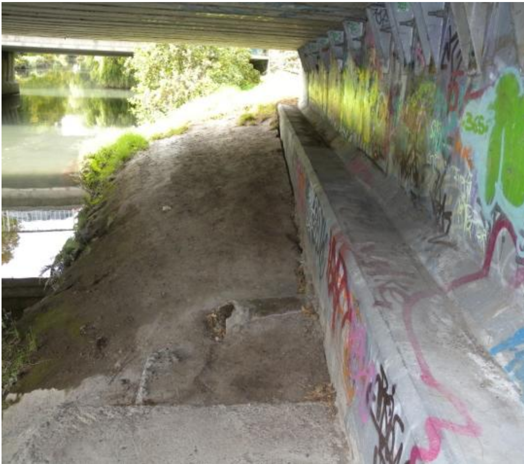
Figure 4.2. Fitzgerald Bridge (B1 on map of Figure 4.1). Performance of southern abutment after Christchurch earthquake. No signs of lateral ground deformation occurred at the southern abutments of the twin bridges. The soil is still attached to the abutment.
