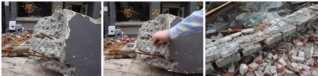
Figure 3.15. Insufficient reinforcement, low quality concrete and bad application caused collapse of a decorative beam and 1 casualty.
