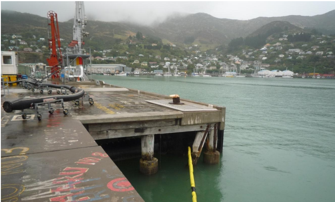
Figure 5.22. Another typical pile configuration (site W3 in the map of Figure 5.6). The concrete piles performed well.
