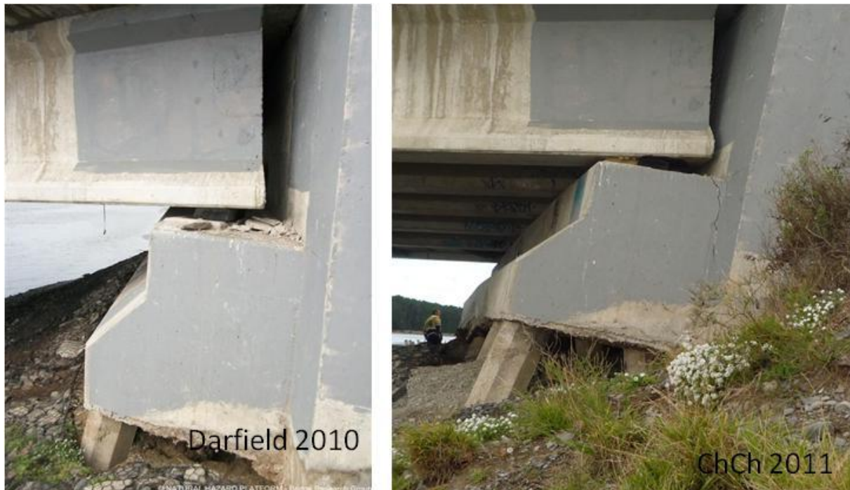
Figure 4.39. Western abutment of South Bridge Road Bridge (B8 on map of Figure 4.1). Differences between Darfield and Christchurch shaking events. After Christchurch earthquake the piles have been more exposed due to greater lateral spreading of the soil and some cracks have been developed in the abutment. Source: NHP- Bridge Research Group.
