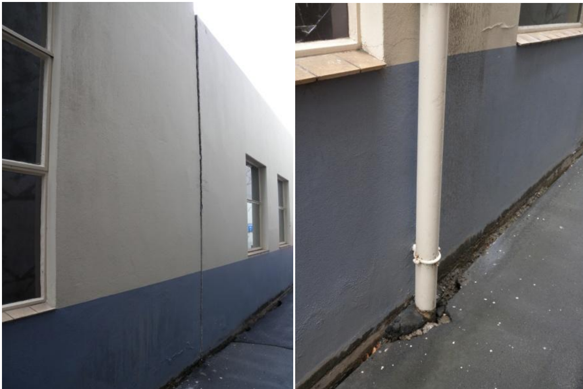
Figure 2.15. Gap between the front and rear section of CHHC seismic station building (left). Liquefied sand was ejected from the crack (right).
