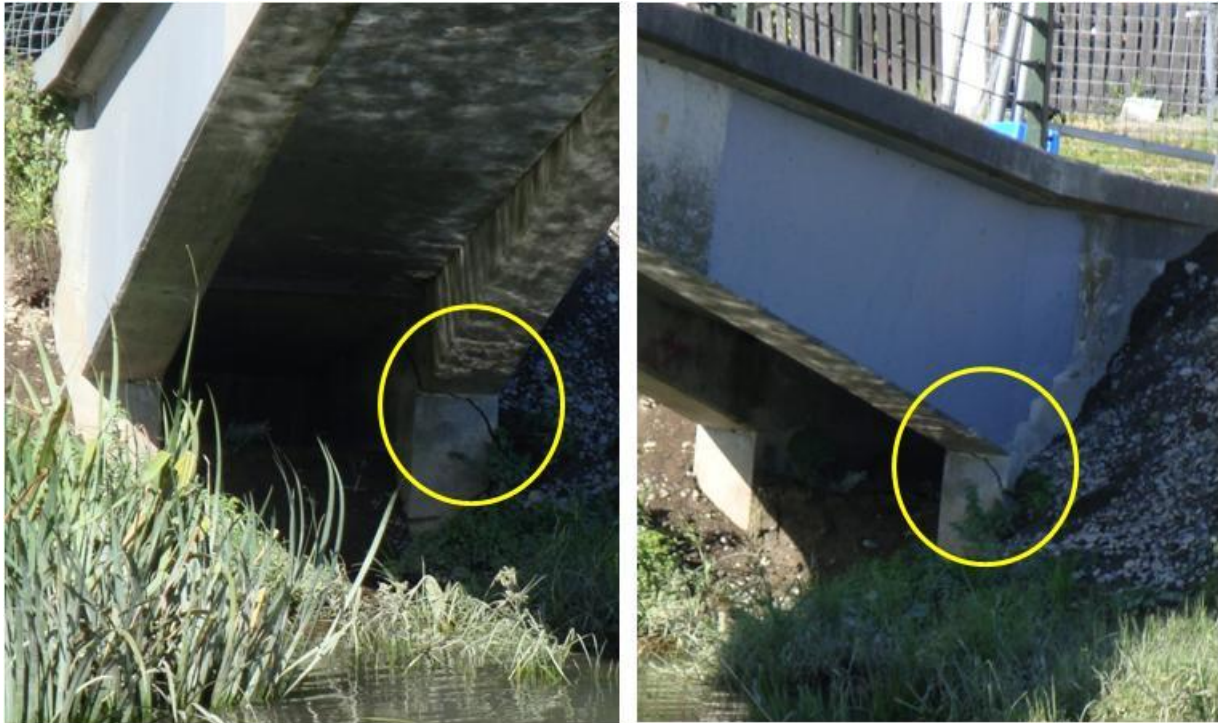
Figure 4.22. Snell Footbridge (B5 on map of Figure 4.1) after Christchurch earthquake. Cracks on the abutments.
