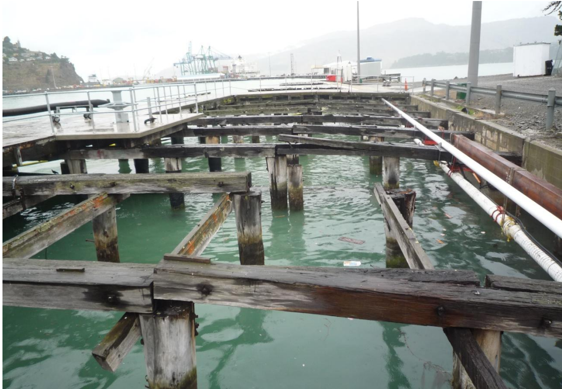
Figure 5.20. Settlement of the backfill caused detachment of the wooden beams from the pile heads (site W3 in the map of Figure 5.6).
