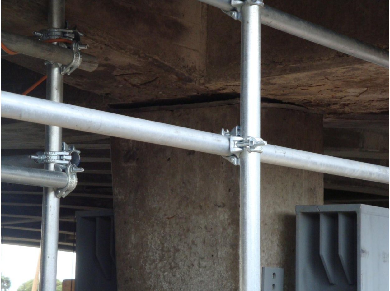
Figure 4.49. West pier of Ferrymead Bridge after Christchurch earthquake (B8 on map of Figure 4.1). The gap opening between the top of the pier and the deck was caused by the inward movement at the base of the pier.
