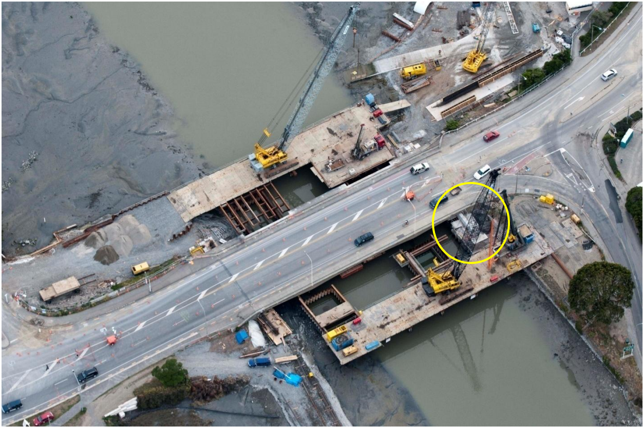
Figure 4.43. Ferrymead Bridge (B8 on map of Figure 4.1). Construction site in the process of strengthening and widening of the bridge. Photo taken after Christchurch earthquake. The new east abutment, in the yellow circle, was built one month before the shaking event.
