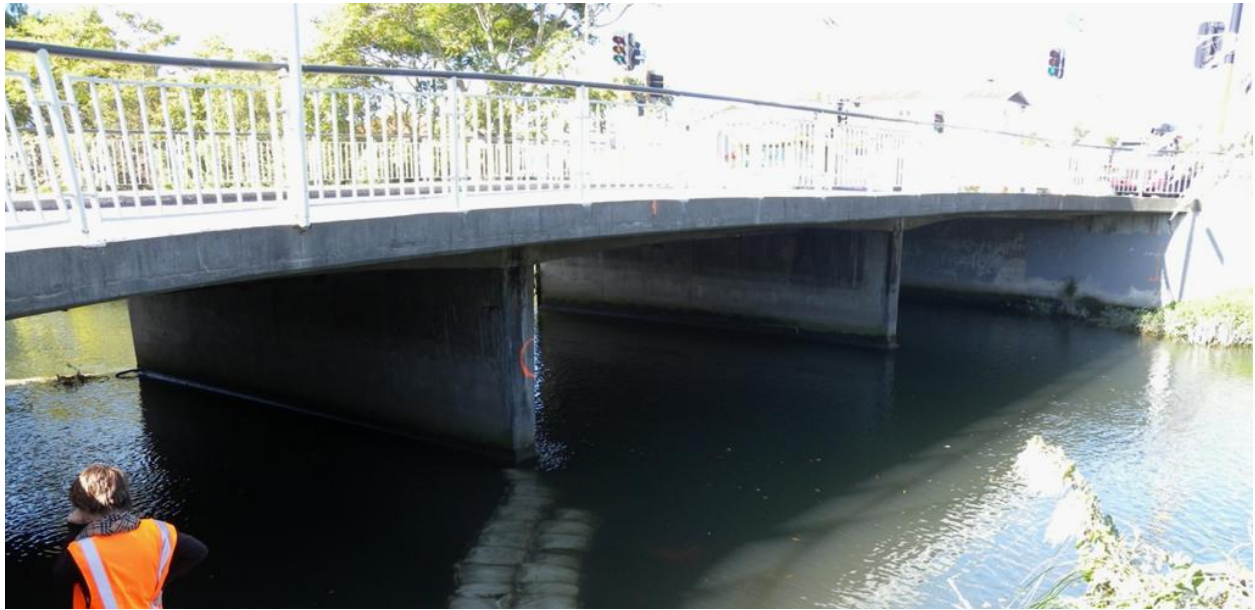
Figure 4.15. Gayhurst Bridge (B4 on map of Figure 4.1) after Christchurch earthquake. The southern abutment appears practically undamaged on the right side of the photo.
