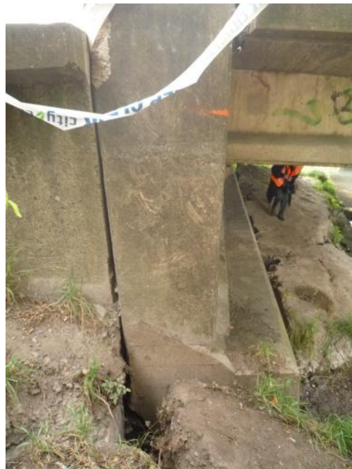
Figure 4.5. Fitzgerald Bridge (B1 on map of Figure 4.1). Performance of northern abutment after Christchurch earthquake. Rotation of abutment is evident due to lateral spreading. The backfill has differentially subsided relative to the abutment.
