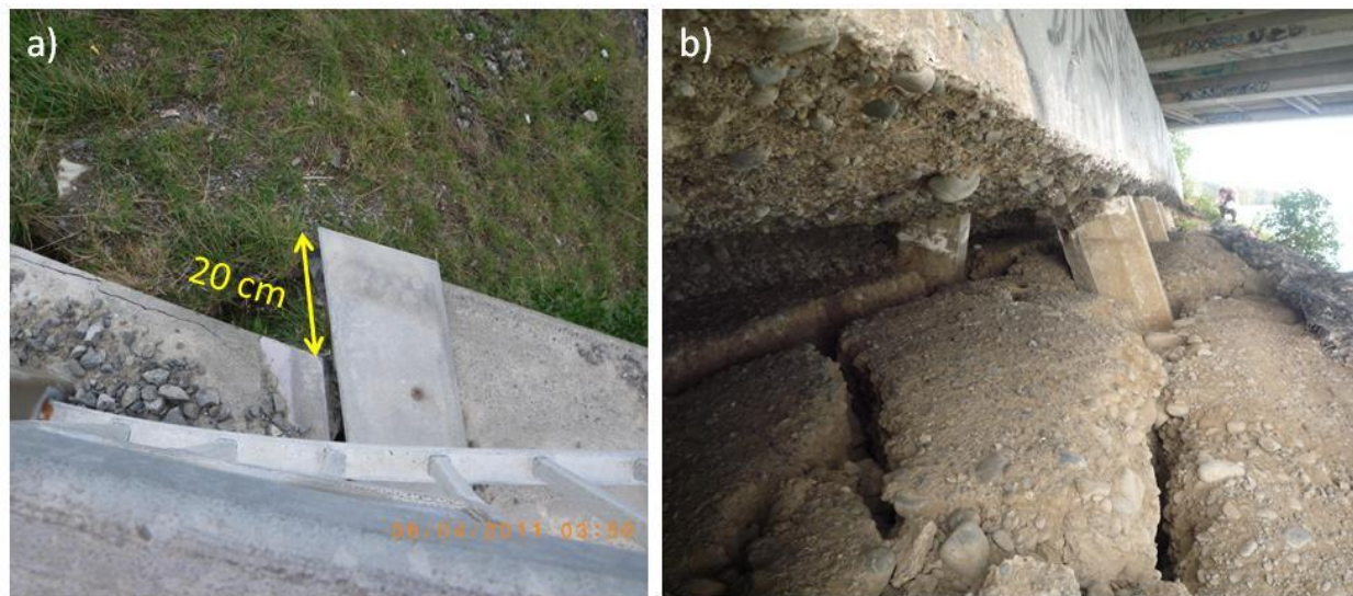
Figure 4.37. Eastern abutment of South Bridge Road Bridge (B8 on map of Figure 4.1) after Christchurch earthquake. a) Differential movement of abutments relative to the deck in the skew line direction is up to 20 cm accumulatively, b) the soil underneath the abutments has moved riverwards opening large cracks in the superficial crust and crating gaps in the front side of the piles.
