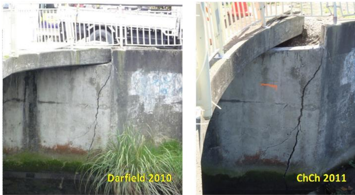
Figure 4.21. Eastern side of the northern abutment of Gayhurst Bridge (B4 on map of Figure 4.1). Comparison of damage between Darfield and Christchurch shaking events. The cracks have widened and the differential lateral riverward displacement of the abutment and wingwalls relative to the deck has increased after Christchurch earthquake. SOURCE.
