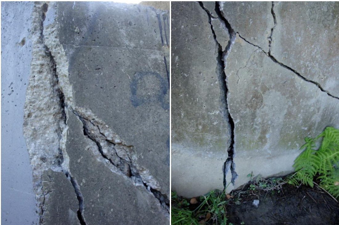
Figure 4.20. Closer look on the cracks of the western wingwall at the northern part of Gayhurst Bridge (B4 on map of Figure 4.1). The cracks have widened and deepened, while concrete spalling had occurred during Christchurch earthquake.
