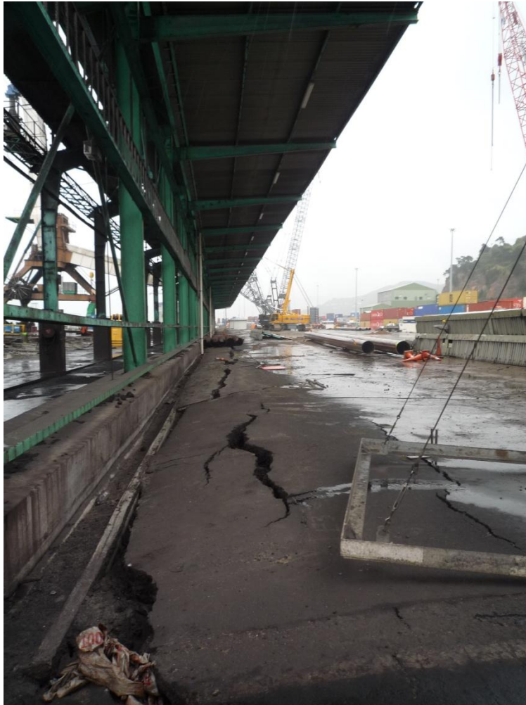
Figure 5.18. Large uniform settlement under the heavy load of the structure. Cracks in the asphalt due to heaving of the ground at right side of the steel structure (site W2 in the map of Figure 5.6)
