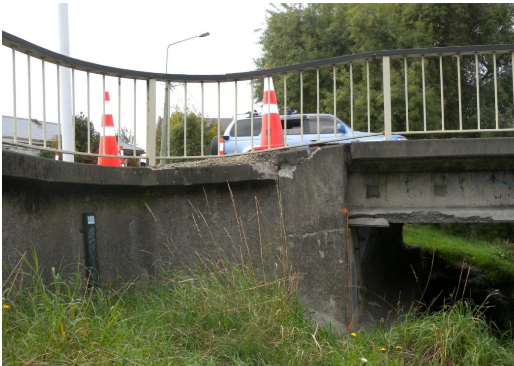
Figure 4.7. Fitzgerald Bridge (B1 on map of Figure 4.1). Performance of northern abutment of the twin bridge after Christchurch earthquake. Rotation of abutment and slump of the backfill occurred. Concrete spalling of the deck developed close to the abutment-seat.
