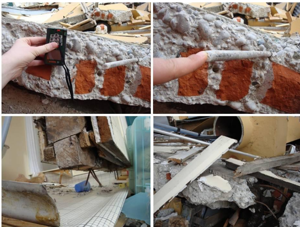
Figure 3.8. The heavy external wall and the slab detail of the collapsed Stonehurst Hostel.
