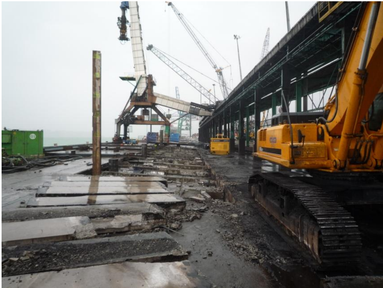
Figure 5.19. Detachment of the slabs of the platform due to differential settlement (site W2 in the map of Figure 5.6). Now the slabs have been removed from their initial place.
