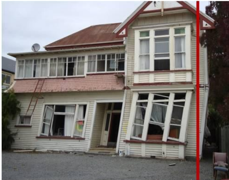
Figure 3.6. Collapsed wooden residence at Gloucester St.
