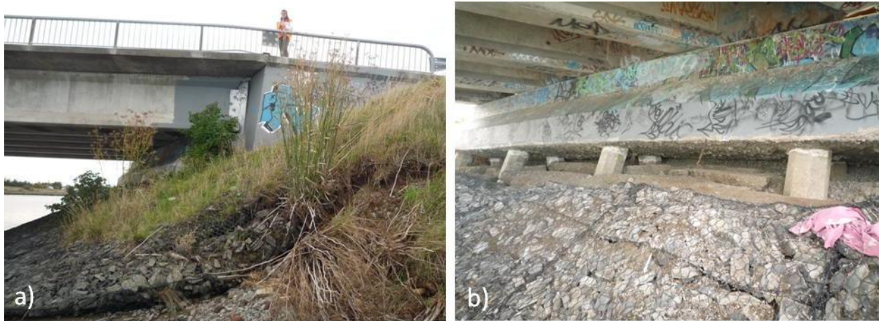
Figure 4.36. Eastern abutment of South Bridge Road Bridge (B8 on map of Figure 4.1) after Christchurch earthquake. a) Back rotation of the abutment around the deck and slump of the approach fill, b) the soil underneath the abutments has moved riverwards exposing both rows of piles.
