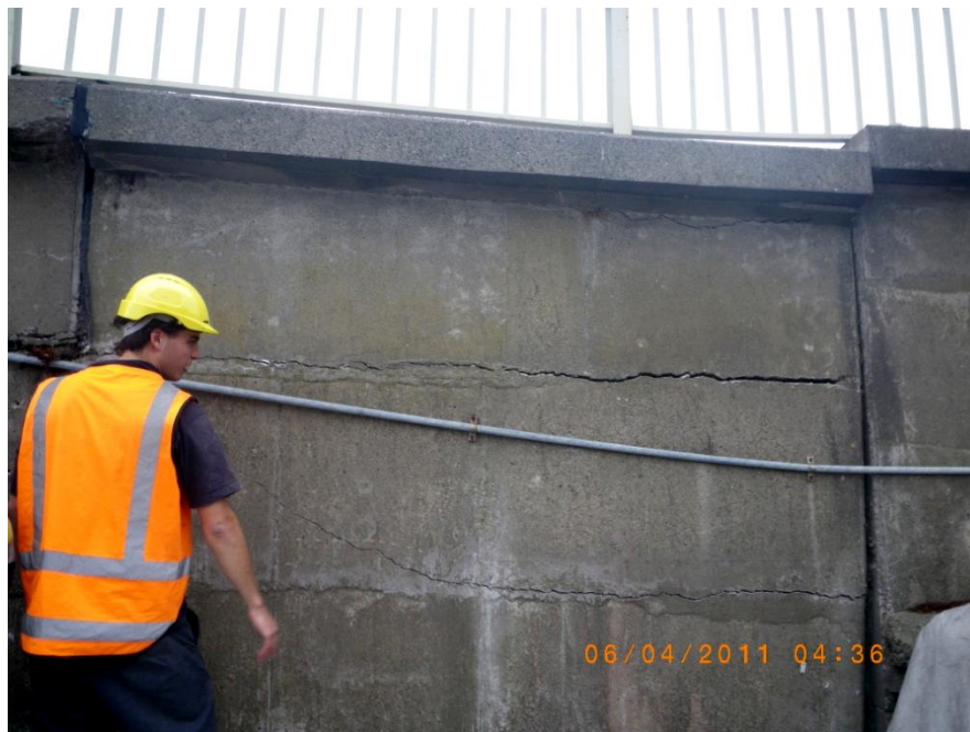
Figure 4.46. East abutment of Ferrymead Bridge after Christchurch earthquake (B8 on map of Figure 4.1). Horizontal cracks in the abutment wall have developed. The major crack is located at the height of the lower part of the deck.
