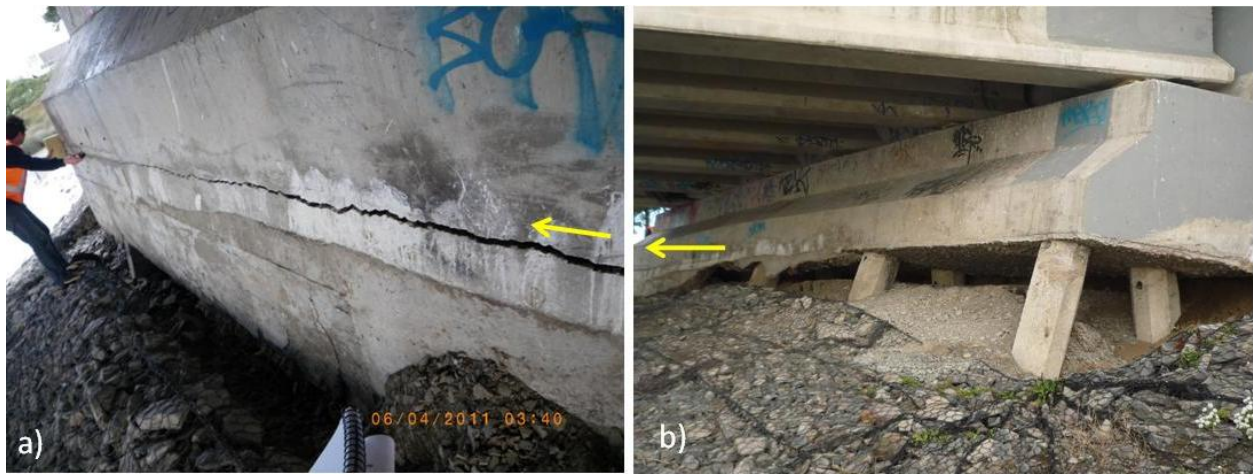
Figure 4.34. Western abutment of South Bridge Road Bridge (B8 on map of Figure 4.1) after Christchurch earthquake. a) Large tension horizontal crack at the base of the abutment, b) The gabion mat used for erosion protection in front of the abutment has laterally and vertically moved so that a great part of the pile heads has been exposed.
