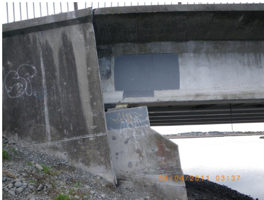
Figure 4.33. Western abutment of South Bridge Road Bridge (B8 on map of Figure 4.1) after Christchurch earthquake. Back rotation of the abutment around the deck and slump of the approach fill.
