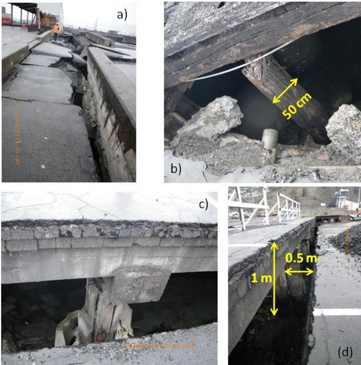
Figure 5.17. Damage of the container terminal quay (site W2 pointed in the map of Figure 5.6): a) Crack opening and distortion of the asphalt connecting the terminal with the wharves, b) Plastic hinging at the top of a timber pile of 50 cm diameter, c) Relative movement of the deck to the pile, d) Separation of the wharf to the backfill due to 1 m settlement of the backfill and outward movement of the wharf up to 50 cm.
