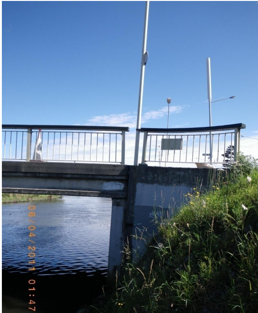
Figure 4.28. Northern abutment of Avondale Bridge (B6 on map of Figure 4.1) after Christchurch earthquake. Moderate back rotation (4 degrees) with only slight settlement of the backfill.
