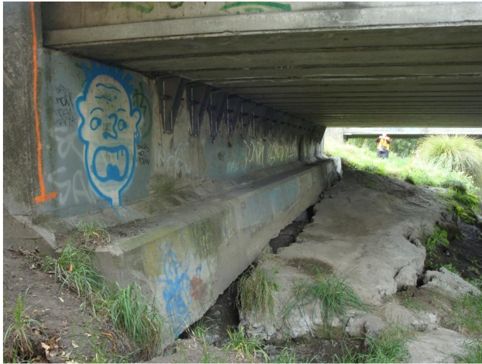
Figure 4.4. Fitzgerald Bridge (B1 on map of Figure 4.1). Performance of northern abutment after Christchurch earthquake. Lateral spreading of the ground has exposed the pile heads.
