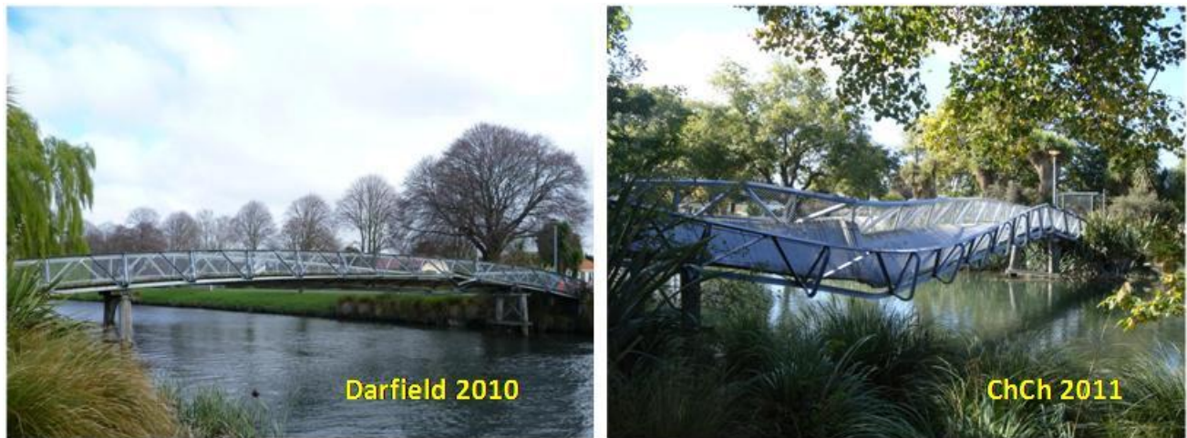
Figure 4.14. Medway Pedestrian Bridge (B3 on map of Figure 4.1). Comparison of bridge damage between Darfield and Christchurch earthquakes. Source: NHP- Bridge Research Group.
