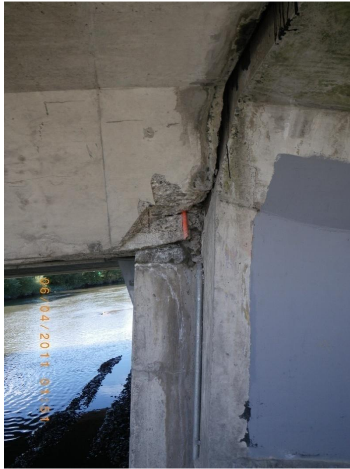
Figure 4.26. Southern abutment of Avondale Bridge (B6 on map of Figure 4.1) after Christchurch earthquake. Concrete spalling and gap opening at the joint of the deck with the abutment.
