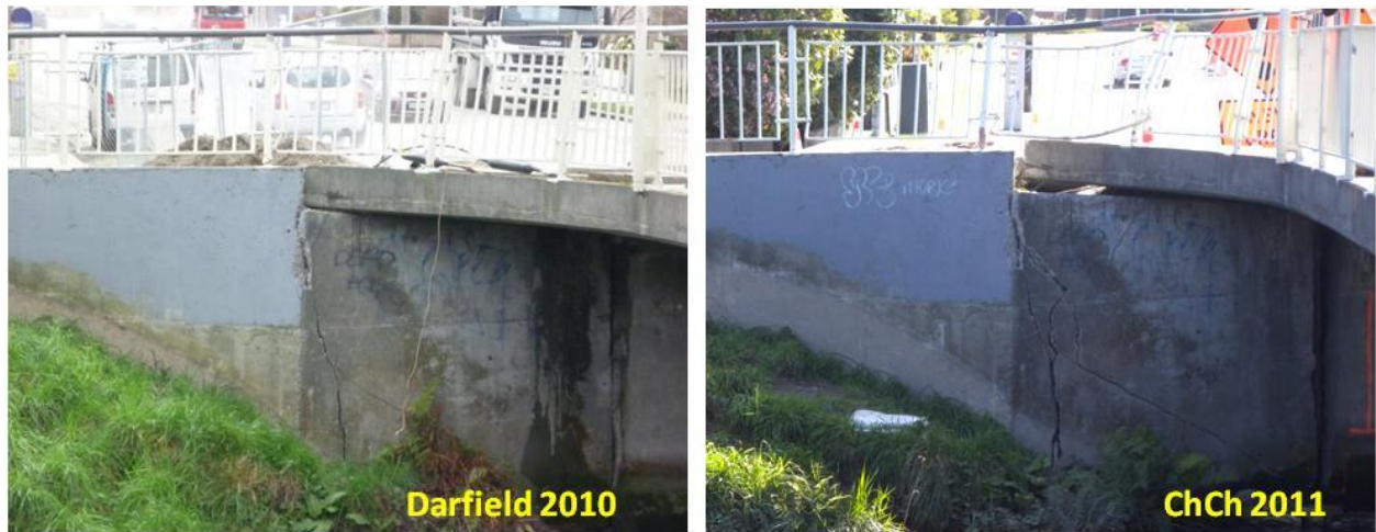
Figure 4.19. Western side of the northern abutment of Gayhurst Bridge (B4 on map of Figure 4.1). Comparison of damage between Darfield and Christchurch shaking events. The cracks have widened and extended, while the differential lateral riverward displacement of the abutment and wingwalls relative to the deck has increased after Christchurch earthquake. Source: NHP-Bridge Research Group.
