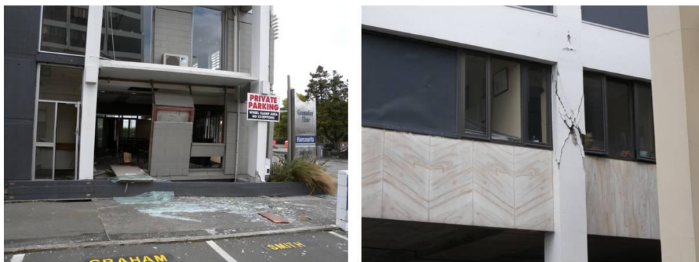
Figure 3.25. Heavily damaged buildings at Madras Street.
