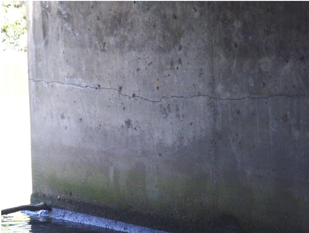
Figure 4.16. Gayhurst Bridge (B4 on map of Figure 4.1) The pier wall close to the northern abutment developed horizontal tension cracks, about 1 m below the deck due to intense shaking and lateral spreading.
