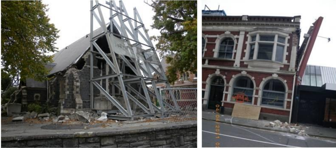
Figure 3.16. Out-of-plane failures around Hereford Street.
