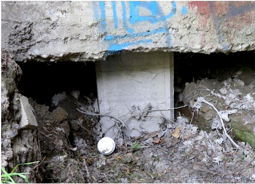
Figure 4.6. Fitzgerald Bridge (B1 on map of Figure 4.1). Rotation of northern abutment has caused tension cracks at the pile-tops.
