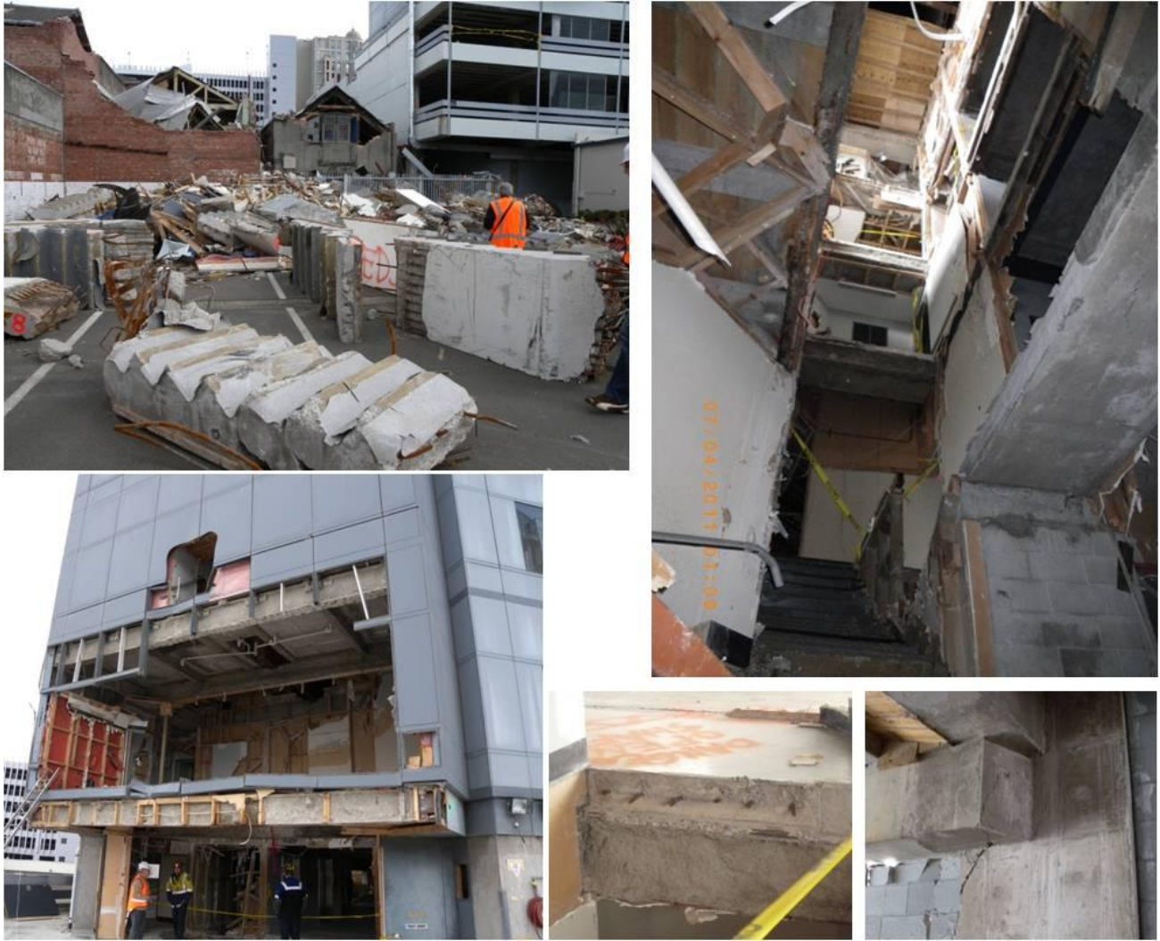
Figure 3.30. Damage in the Forsyth Barr Building and its collapsed stairs.
