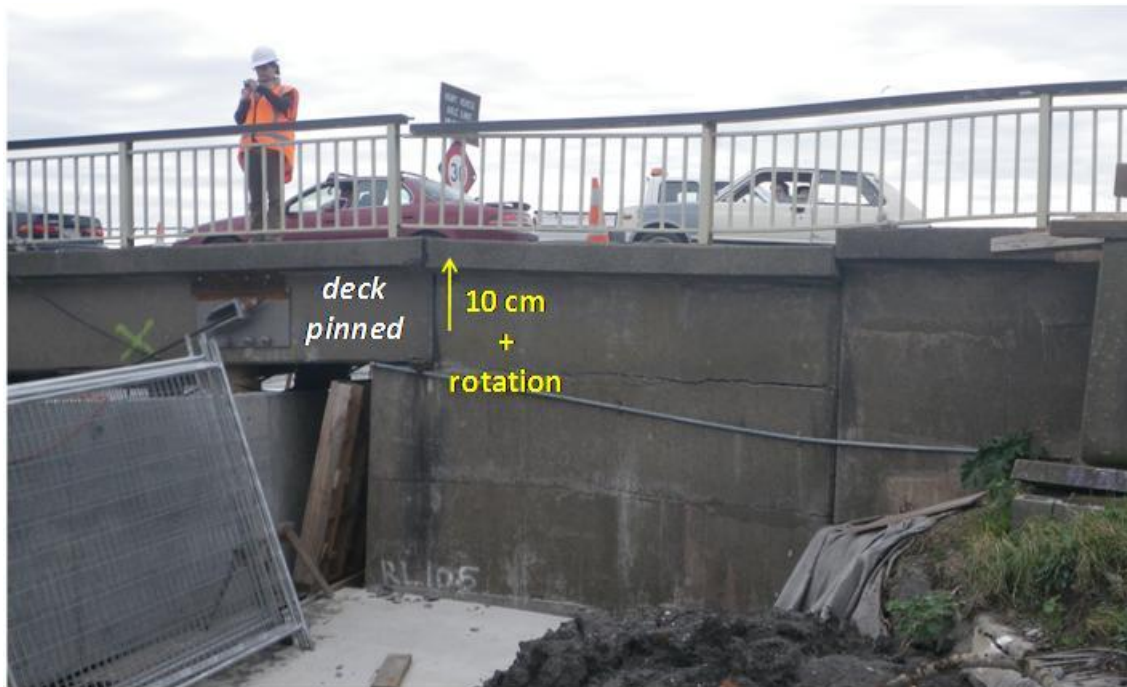
Figure 4.45. East abutment of Ferrymead Bridge after Christchurch earthquake (B8 on map of Figure 4.1). The front section of the abutment has back rotated and moved upwards by 10 cm. The rear section of the abutment has been displaced in a similar trend.
