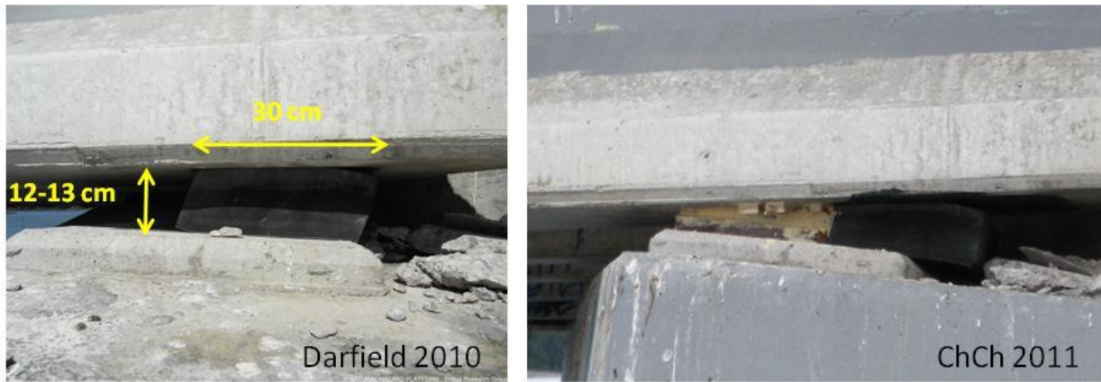
Figure 4.38. Western abutment of South Bridge Road Bridge (B8 on map of Figure 4.1). Differences between Darfield and Christchurch shaking events. The rubber bearing pad had sheared and slid laterally in Darfield earthquake. After Christchurch earthquake the rubber pad has deformed and displaced even more. The timber pad, used as a stop probably has been placed after Darfield earthquake, because it seems to have sustained certain deformation. Source: NHP- Bridge Research Group..
