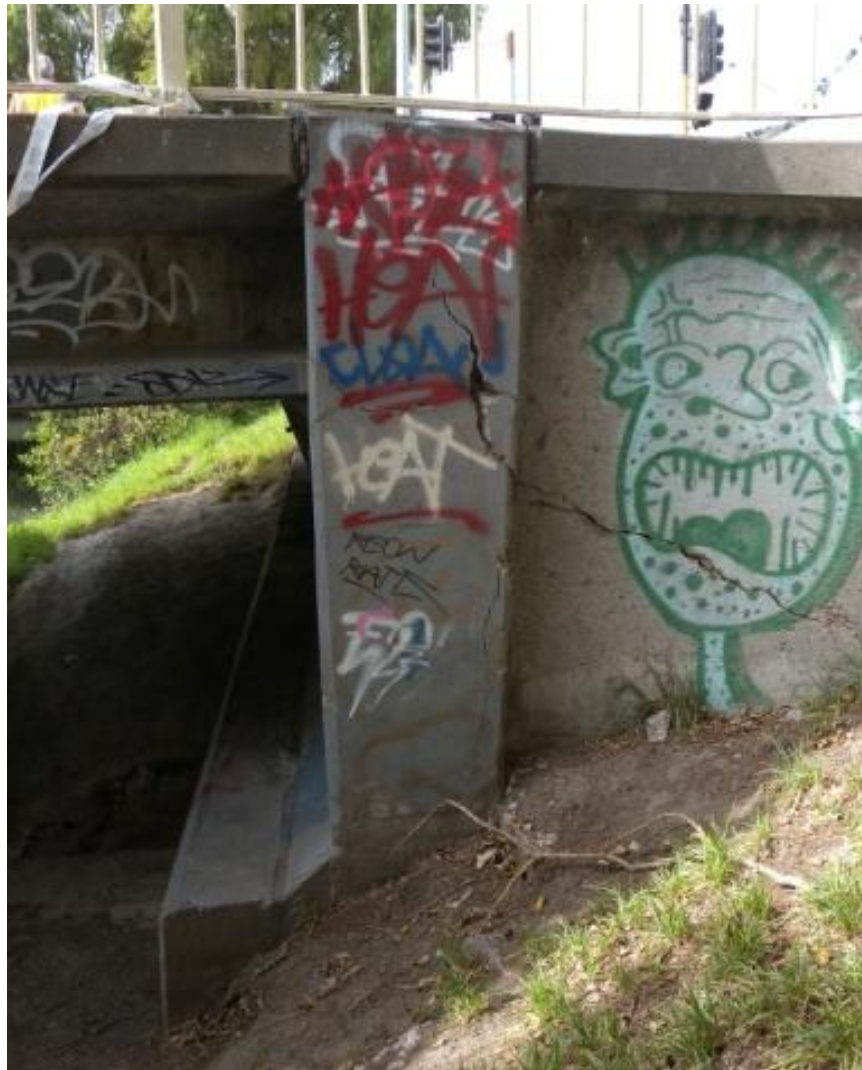
Figure 4.3. Fitzgerald Bridge (B1 on map of Figure 4.1). Performance of southern abutment after Christchurch earthquake. No lateral ground deformation occurred at the southern abutments of the twin bridges. Thus, there was no rotation of the abutment. However, the abutment suffered moderate cracks due to seismic and inertial load.
