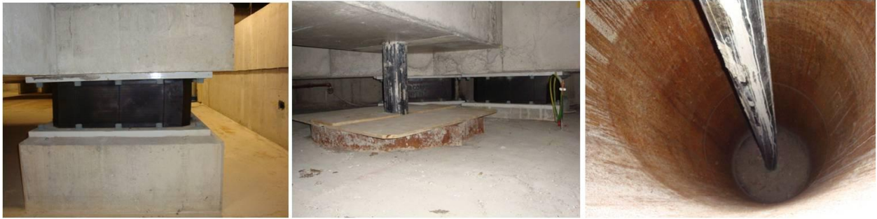
Figure 3.42. Rubber bearing (left) and the restraining ground anchorage.
