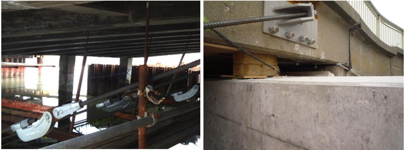
Figure 4.47. East abutment and pier of Ferrymead Bridge after Christchurch earthquake (B8 on map of Figure 4.1). The base of the piers has been tied with tendons to the edges of the deck in order to keep and restrain any inward movement (left). Timber pads have been placed between the new abutment and the deck after the earthquake (right).
