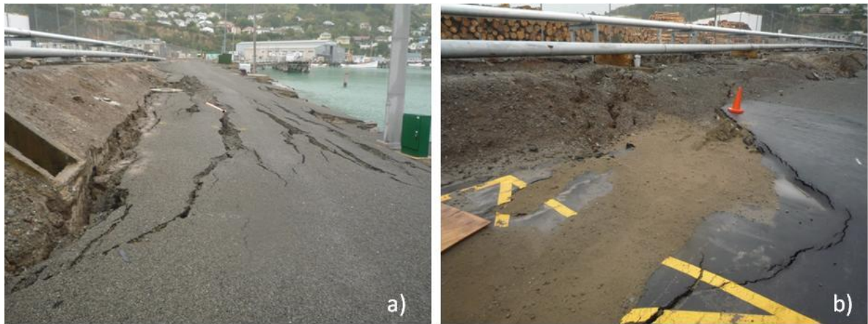
Figure 5.25. a) Cracks in the inclined asphalt due to lateral spreading, b) Ejected sand appeared on the surface indicating that liquefaction has occurred (site W3 in the map of Figure 5.6).
