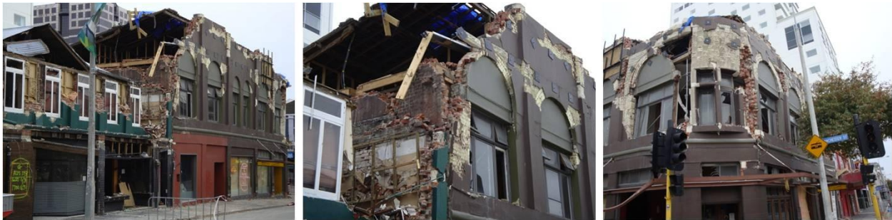
Figure 3.4. Damaged buildings at Manchester Street.
