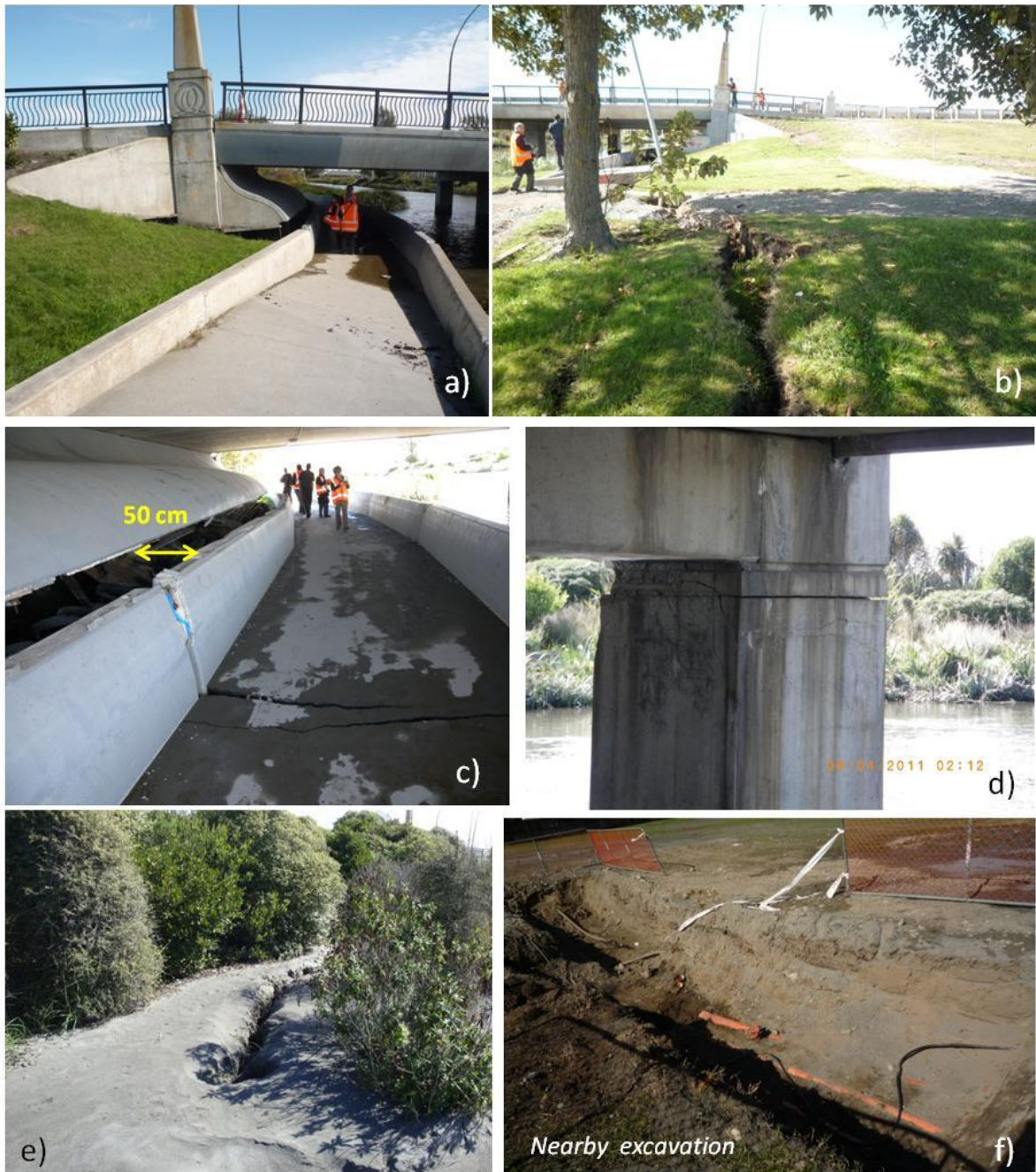
Figure 4.29. Avondale Bridge (B7 on map of Figure 4.1) after Christchurch earthquake. a) Back rotation of the abutments and slump of the approach fill, b) Large lateral spreading cracks in the ground parallel to Avon river coast extending in a great distance from the abutments indicating horizontal ground displacement more than 1, c) Riverward ground displacement in front of the abutments forming a gap of 50 cm, exposing the top of the piles, d) Concrete spalling and cracks at the top of the pier-column due to intense shaking and lateral spreading, e) Significant quantity of sand ejecta close to the bridge, f) Nearby shallow excavation shows a top crust of clay containing thin beds of sand.
