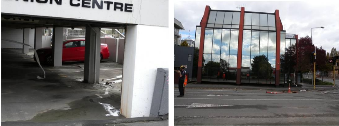
Figure 3.24. Buildings (B20 left and B22 right) damaged due to differential settlements induced by liquefaction.
