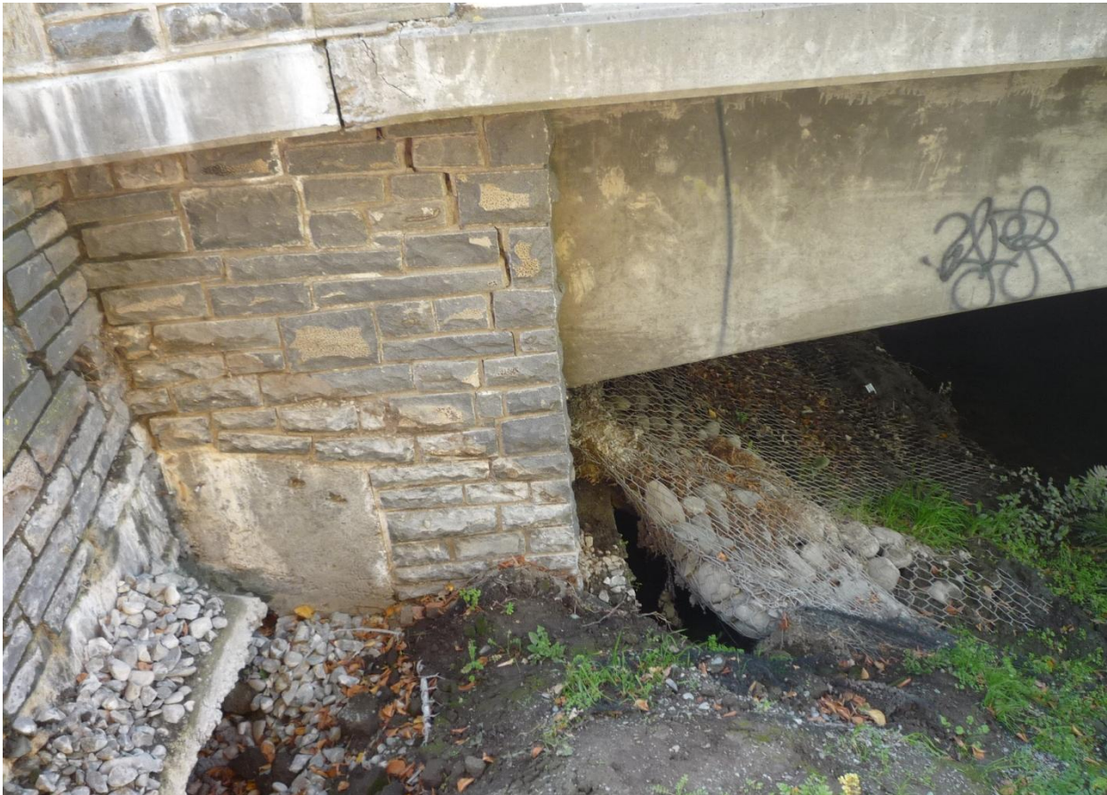
Figure 4.13. Stanmore Bridge (B2 on map of Figure 4.1). Cracks in the abutment and concrete spalling close to the joint with the deck. Gap opening between the abutment and the soil, tending to expose the foundation.
