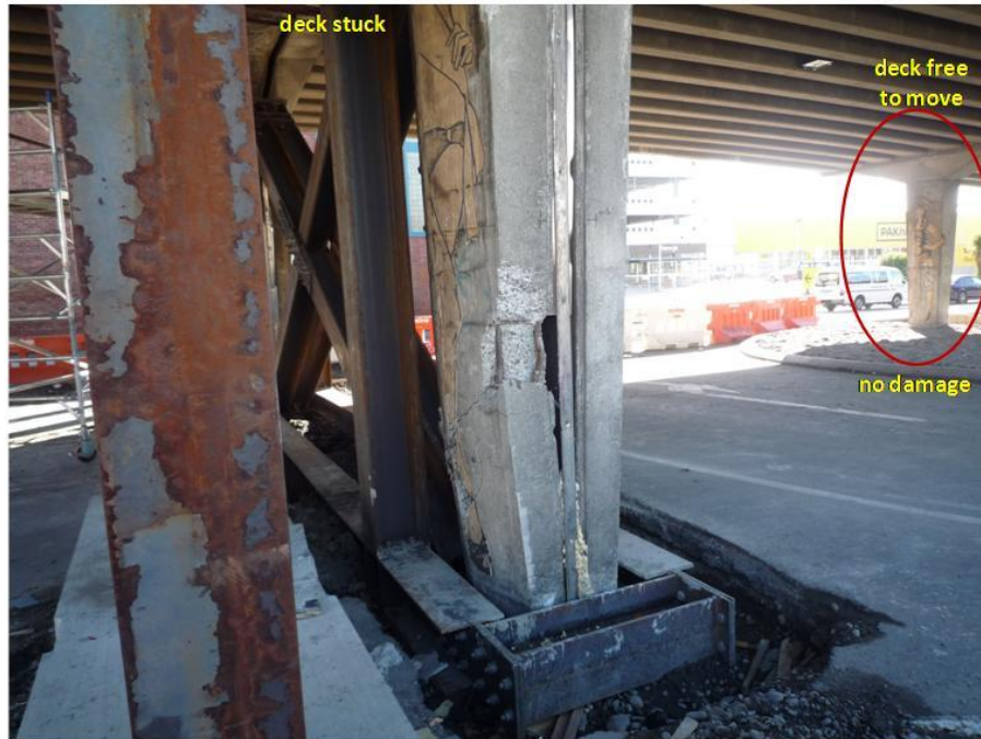
Figure 4.52. Failure of the pier due to shear and then buckling of the rebar under axial loads.
