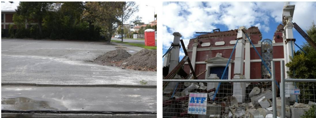
Figure 3.26. Sand boils after liquefaction and collapsed masonry structure at Madras Street.
