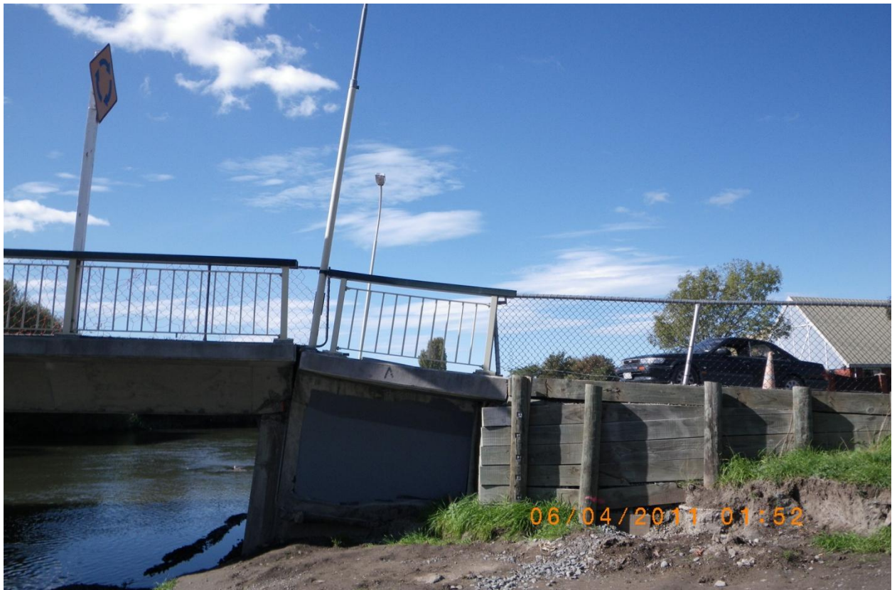
Figure 4.25. Southern abutment of Avondale Bridge (B6 on map of Figure 4.1) after Christchurch earthquake. Back rotation of the abutment (8 degrees) and subsidence of the backfill.
