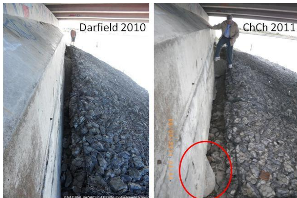
Figure 4.41 Western abutment of South Bridge Road Bridge (B8 on map of Figure 4.1). Differences between Darfield and Christchurch shaking events. After Christchurch earthquake, the lateral soil movement was at least twice as much as in Darfield earthquake. Thus the piles even more exposed. Source: NHP- Bridge Research Group.
