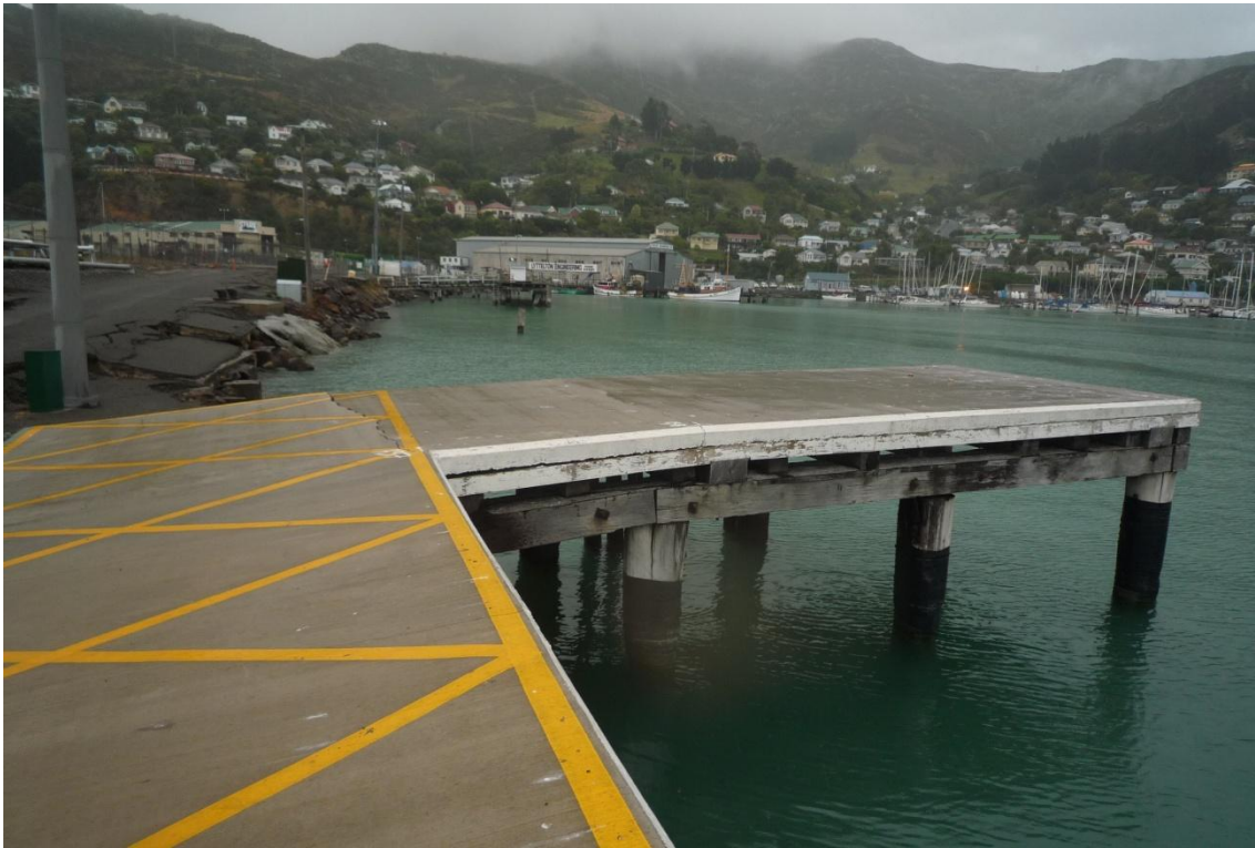
Figure 5.21. One typical pile configuration (site W3 in the map of Figure 5.6). The timber piles have cracked at the top.
