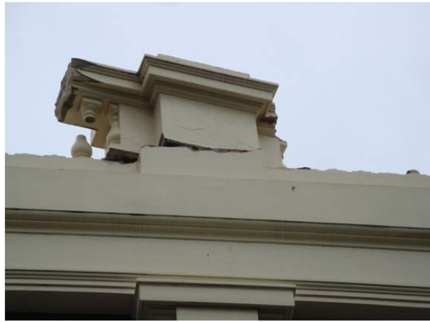
Figure 3.14. Massive decorative element disconnected from the main body of the structure.
