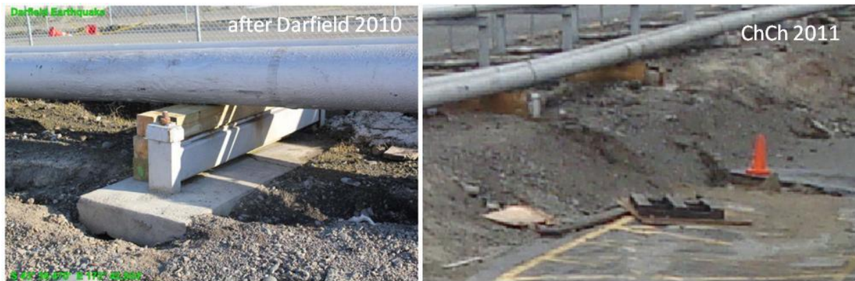
Figure 5.27. Comparison of the fuel pipe line deformation (site W3 in the map of Figure 5.6) between Darfield and Christchurch earthquakes. After Darfield earthquake, temporary wooden support was used to accommodate settlement under fuel line (Cubrinovsky et al., 2010). After Christchurch earthquake, the supports are still there and they have settled together with the fuel line. Photograph from Darfield earthquake can be found in Cubrinovsky et al. (2010).
