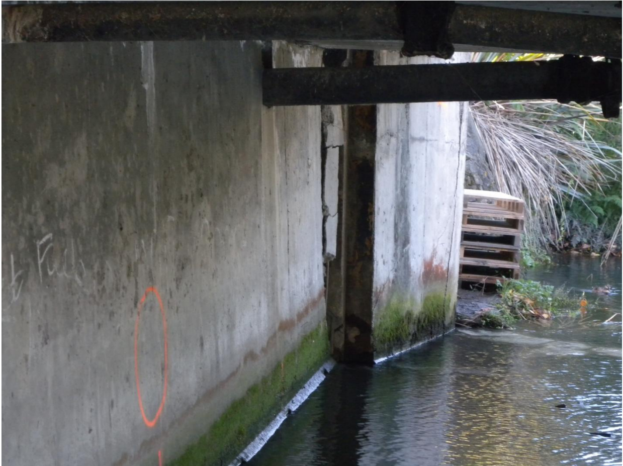
Figure 4.17. Northern abutment of Gayhurst Bridge (B4 on map of Figure 4.1). Rotation and differential riverward displacement (in the order of 70 cm and more) of the eastern wingwall relative to the abutment caused concrete spalling and cracking at the joint of the abutment with the wingwalls.
