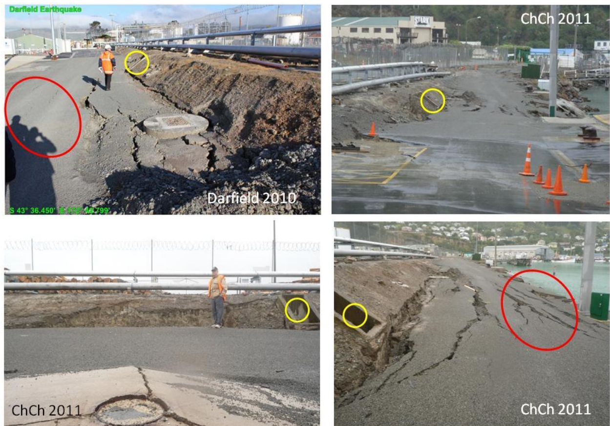
Figure 5.26. Comparison of the damage of site W3 in the map of Figure 5.6 between Darfield and Christchurch earthquakes. The yellow and red circles are the common point of references in all photos. Photograph from Darfield earthquake can be found in Cubrinovsky et al. (2010).
