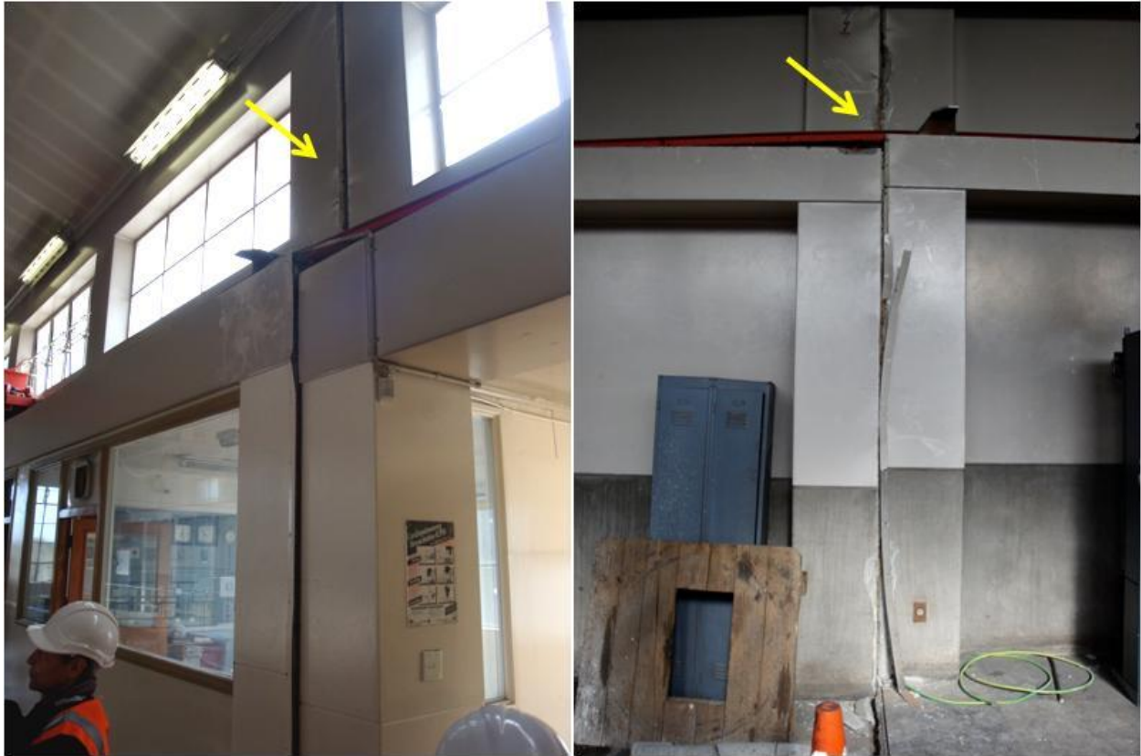
Figure 2.43. Interior of the Pumping Station next to the garage. Differential movement at the joint of one section of the building with the other.
