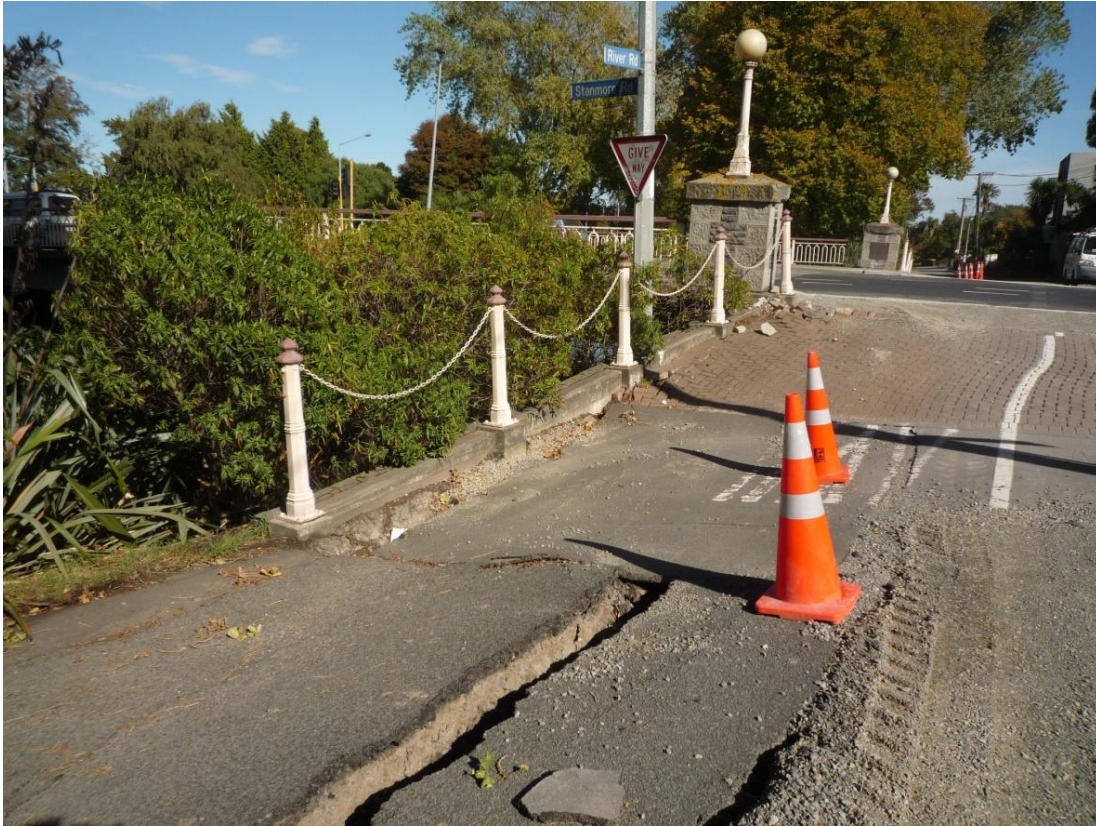
Figure 4.11. Stanmore Bridge (B2 on map of Figure 4.1). Rotation of the abutment around the deck. The street lighting column next to the abutment has rotated riverwards, following the lateral deformation of the ground, while the light column seated on the abutment indicates that the abutment has back rotated due to the deck constraint. Slump of the approach fill is not visible because at the time of our visit, the cracked asphalt between the two abutments had been replaced by new. However the large cracks in the road parallel to Avon river (in the order of 40 cm) due to lateral spreading were still there.
