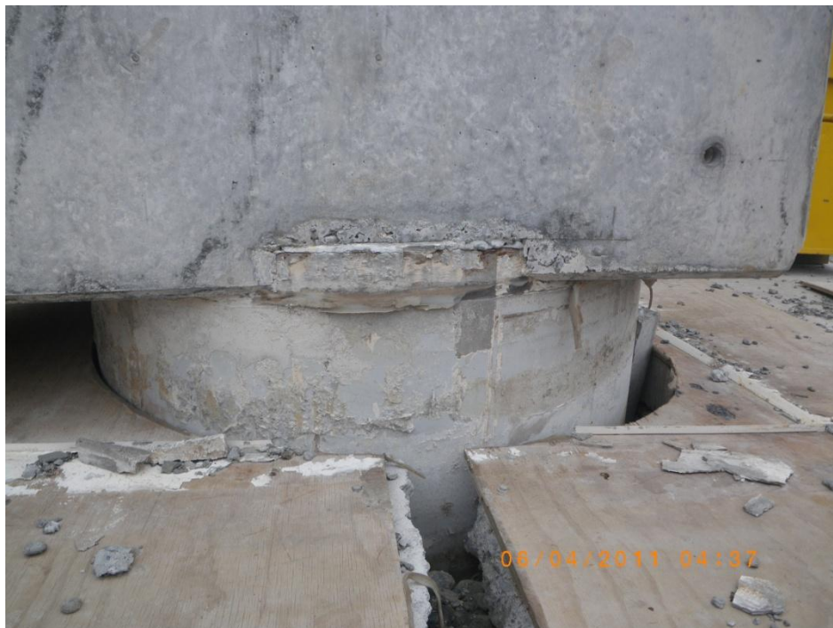
Figure 4.48. New east abutment of Ferrymead Bridge after Christchurch earthquake (B8 on map of Figure 4.1). The abutment has moved towards the center of the bridge. The gap opening at the back side of the pile is a result of this movement.
