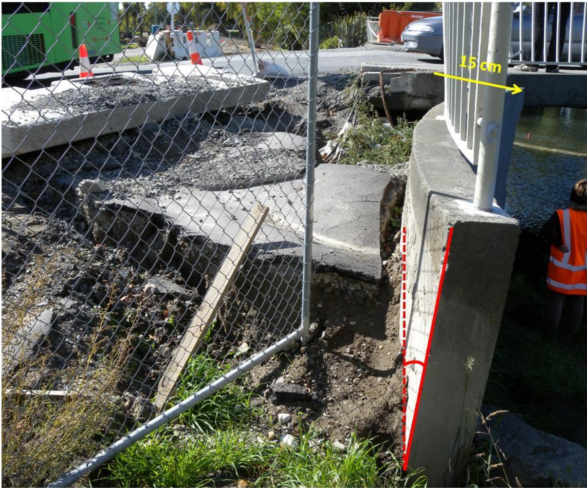
Figure 4.18. Northern abutment of Gayhurst Bridge (B4 on map of Figure 4.1). Rotation and displacement of the western wingwall not only riverwards but also away from the abutment (15 cm approximately at the top) perpendicular to the deck.
